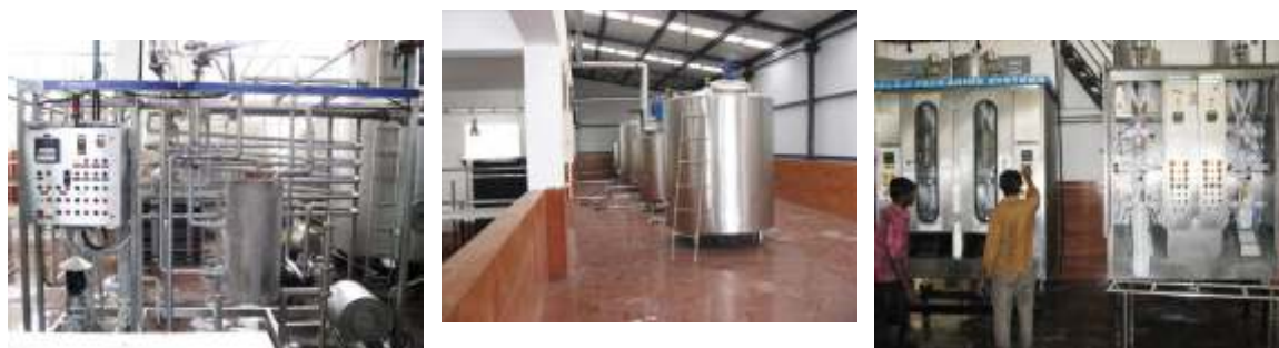
Existing facility at Krishnagiri
